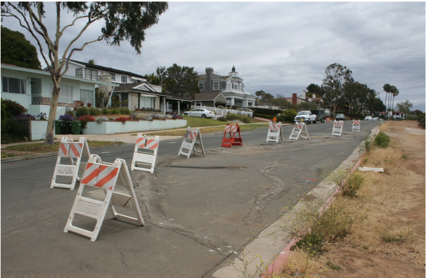
Asilomar Blvd. crown and developing scarp
